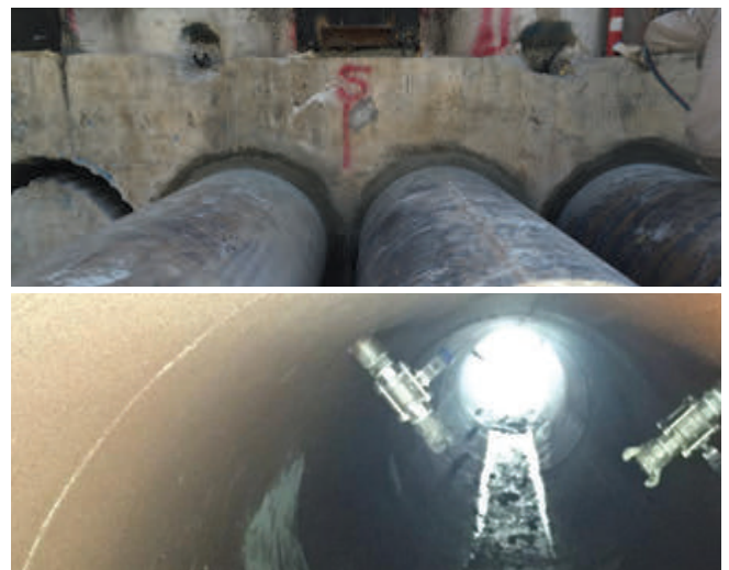
Figure 9: Top: Sealing of the annulus gap between the SBP and the pipe using concrete; Bottom: One-inch ports inside the pipe used to inject bentonite during excavation and annulus grouting
