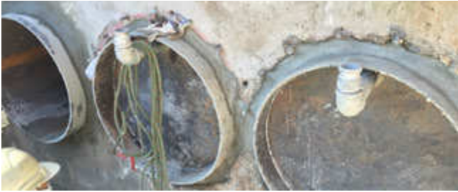
Figure 10: Steel plates were used as end caps for the pipe. Grout was pumped via 2 inch ports welded to the top of the end caps
