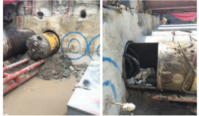
Figure 8: Left: Breakthrough of MTBM at retrieval shaft; Right: Opening for disconnection of umbilical hoses and slurry lines
