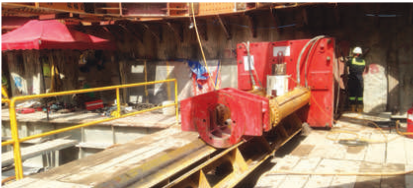
Figure 5: The setup of the jacking frame had to be done for each individual drive
