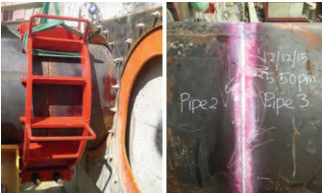
Figure 7: Left: Clamping fixture to ensure concentricity of pipes before welding; Right: DPI testing on completed welds
