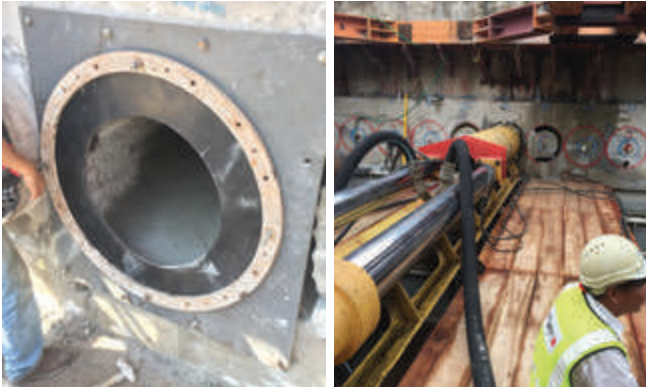
Figure 6: Left: Installed launch shield with rubber gasket; Right: MTBM being launched in the cored SBP
