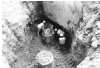
Figure 4b: Jet grouting surrounding excavation for the construction of transfer slab for pile underpinning (after Boon et al., 2015)
