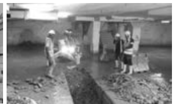
Figure 7: Pre-cutting of existing basement slab, to enable D-wall work to proceed at Pasar Seni Station
