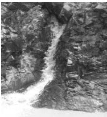
Figure 19: High seepage flows through localised open joint (surrounded by massive limestone with tight joints) that has eluded treatment
