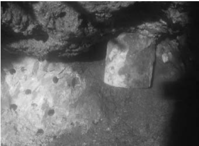
Figure 32: Photo showing API pipe (micropile) encroaching into tunnel horizon
