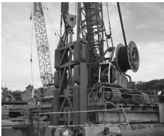
Figure 5: 'Trench Cutter' D-wall machine at Pasar Seni Station sitting on Temporary platform
