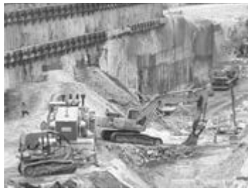
Figure 13: Excavation works at Pasar Rakyat in rock showing - Combination of Drill & Blasts method and Surface Miner
