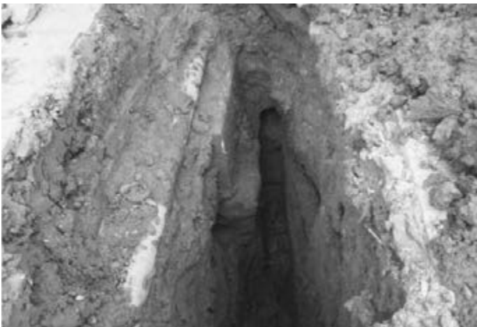
Figure 29: Trial pit to detect size of foundation and type of piles
