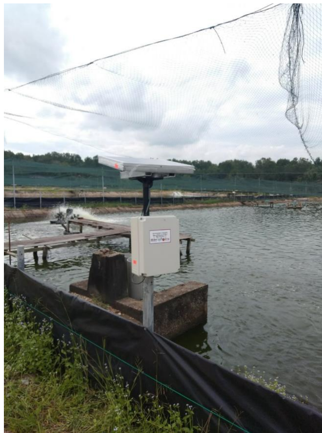
Figure 2. The installed smart aquaculture monitoring system
