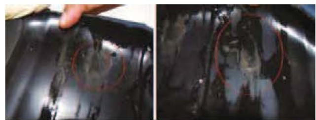
Figure 4: Burn mark at the insulation (B-phase).
