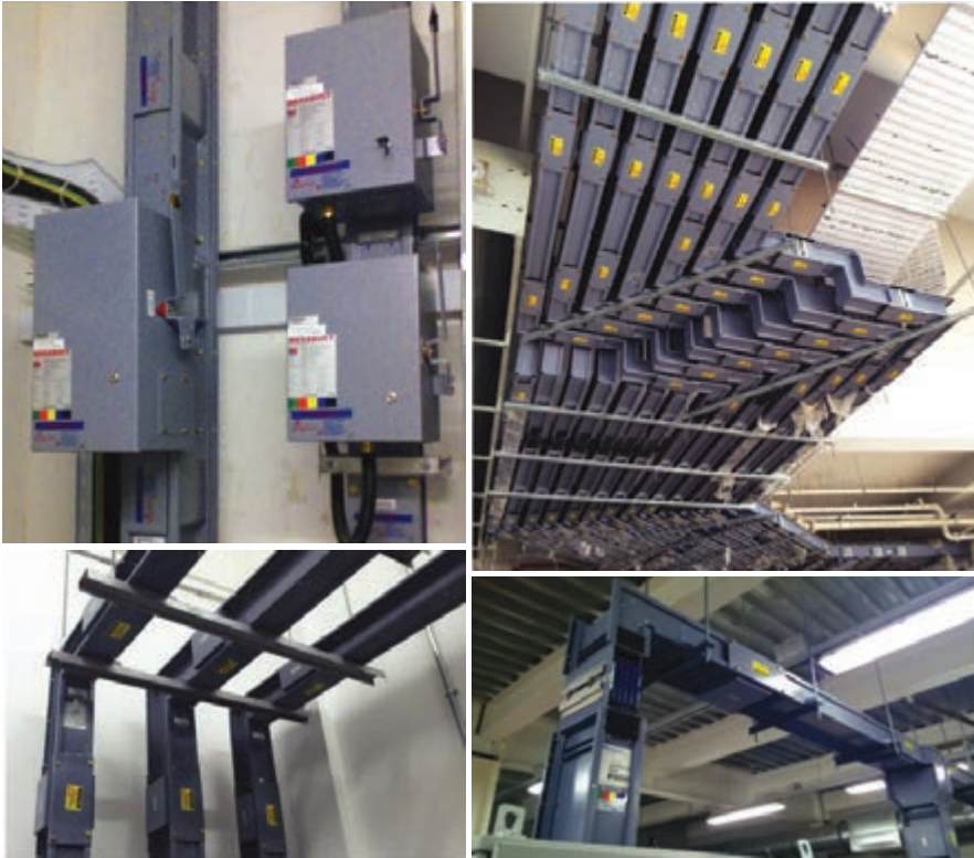
Example of Operating Busduct
