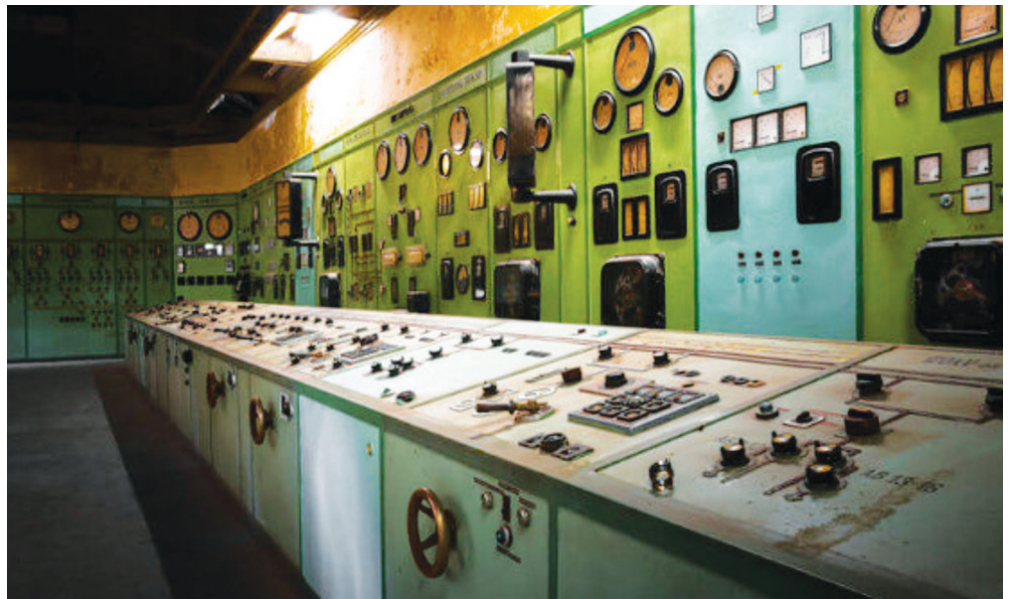
Typical control room
