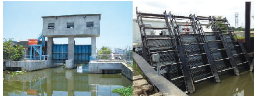
Photo 14: Gate, Trash Rack & Screens
